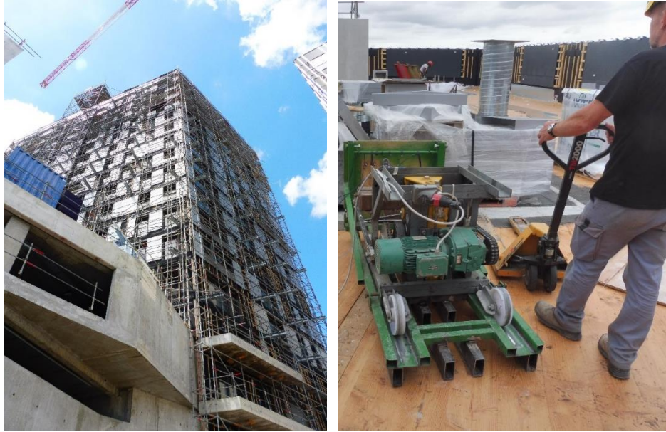
Figure 1. A view of Hyperion building at the time of testing and the shaker on top of the building, ready to operate
